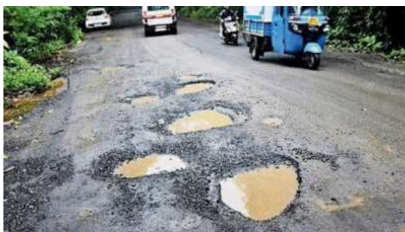
FIGURE 1(a): MULTIPLE POTHOLES
